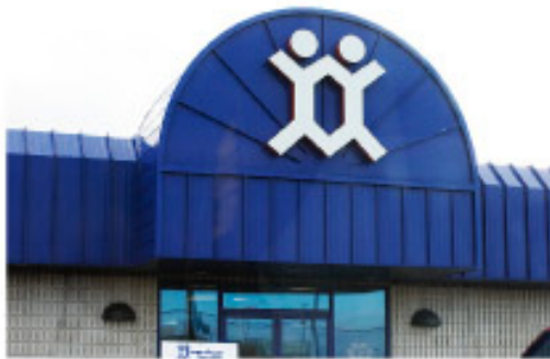
Front fascia system and barrel canopy. Design assistance, fabrication and supply by A G Bell for Zumbrun Construction, Fort Wayne
