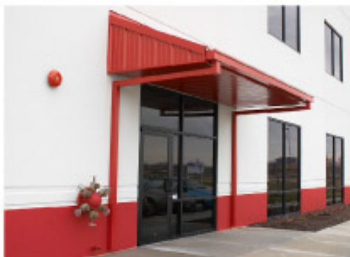
Canopy framing and sheeting by A G Bell installed on a commercial warehouse building in Plainfield, IN by Allied Handling & Equipment, Franklin, IN
